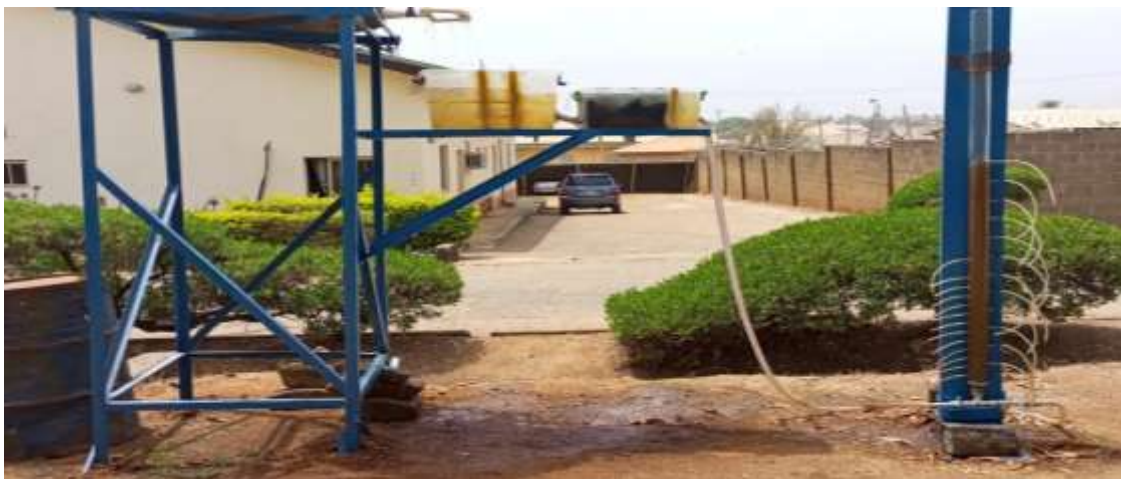
Figure 3; Constructed iron removal pilot model plant
